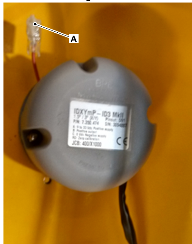
A Spare cable
